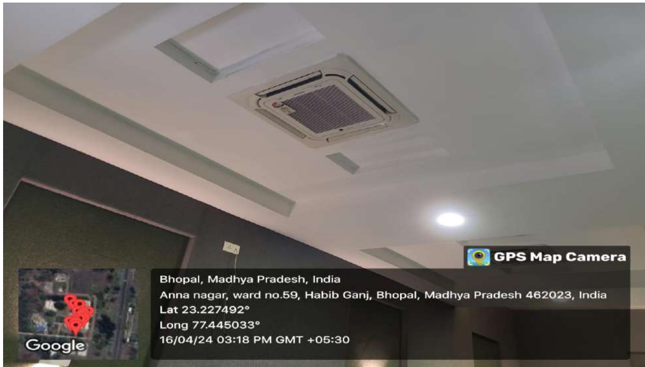
3 Star rated Air Conditioner in Auditorium
